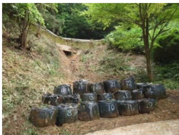
▲被災箇所①
